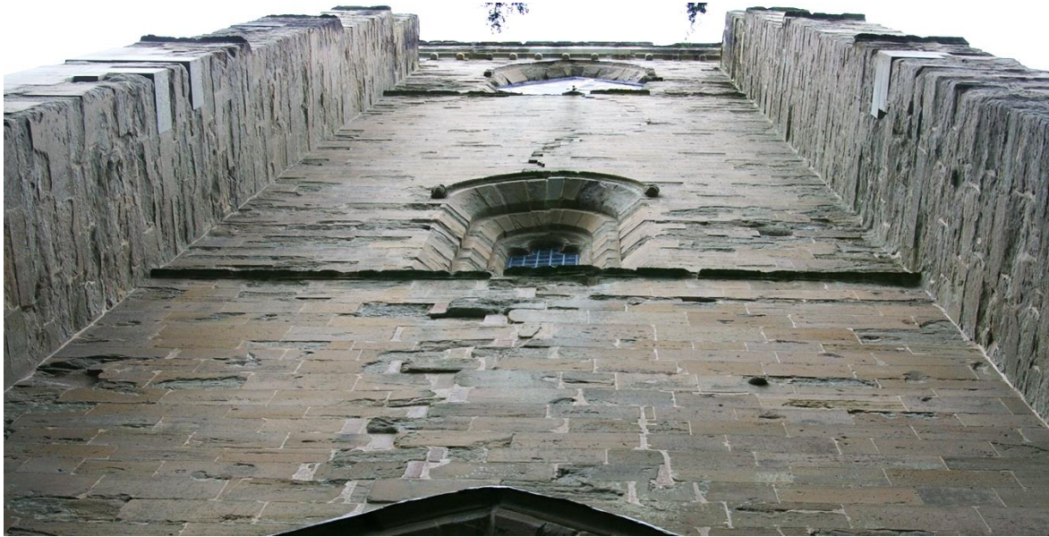
Dunkeld Bell Tower 1452-75: Structural disturbance in consequence of bellringing
