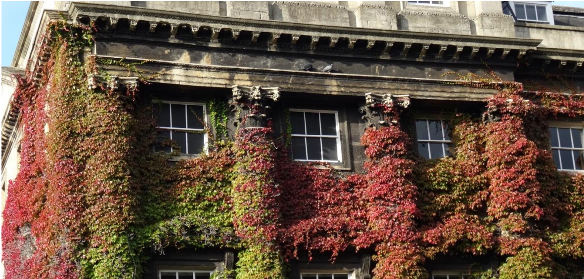
Unrestrained surface growth can obscure possible underlying issues
