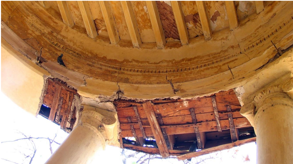
Residency, Hyderabad 1805: A consequence of unrestrained water penetration
