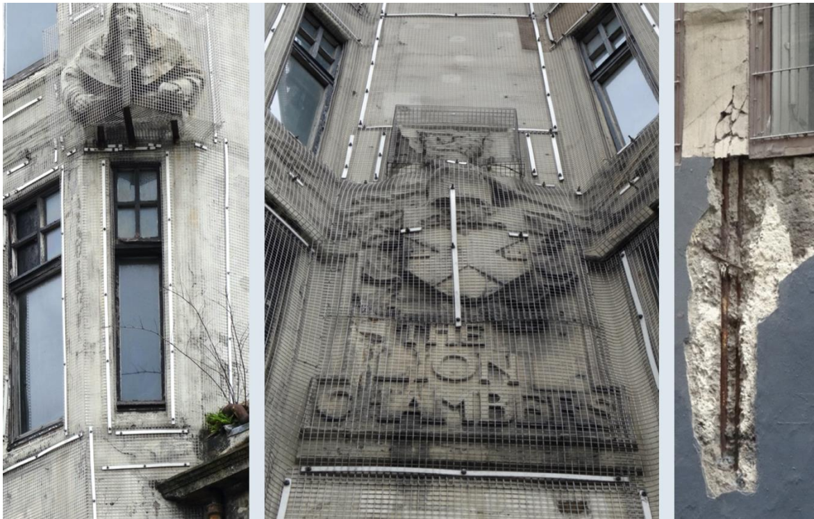
Lion Chambers Glasgow: Spalling concrete surfaces are netted for public safety
