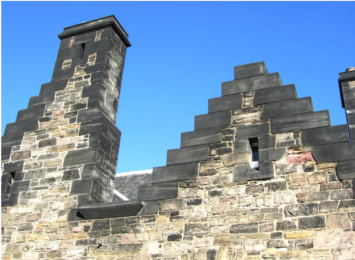
Edinburgh: Variations in surface soiling related to the juxtaposition of different sandstones
