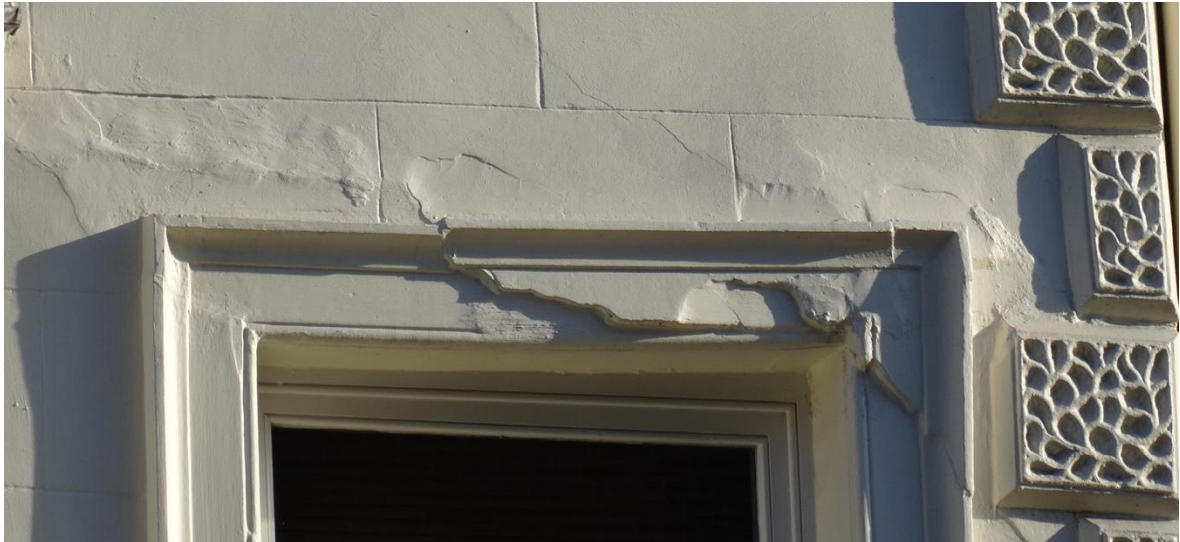
Disguised structural concerns will continue to exist and, most likely, get worse
