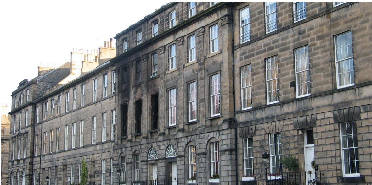
Edinburgh: Georgian property interior lost to fire with external masonry damage
