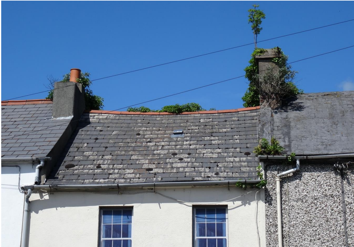
Newtownards: Basic repair needs require timely awareness and action
