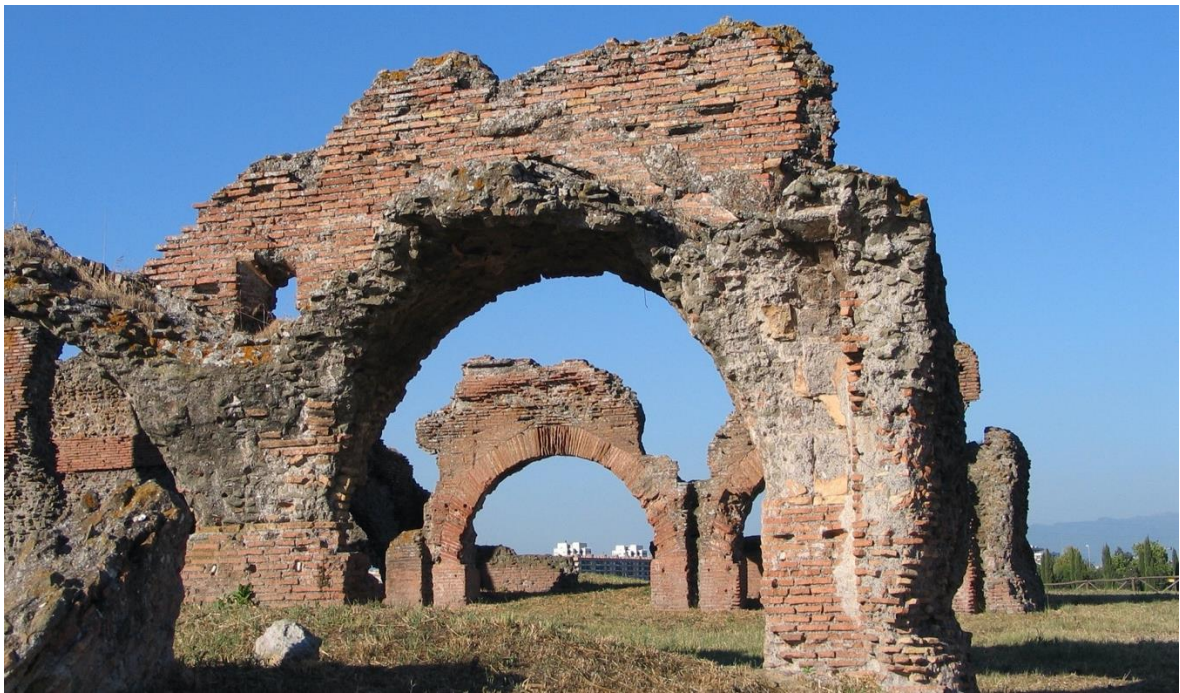
With due care and cost, structural elements can be consolidated and stabilised 'as found'
