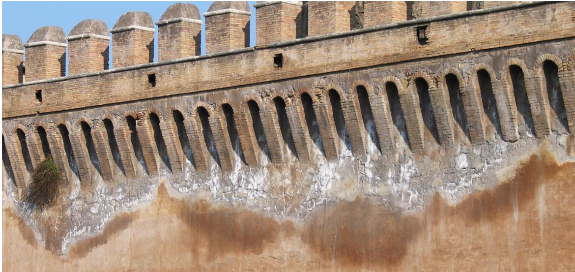
Rome: Diluted salt penetration and efflorescence from a parapet walkway
