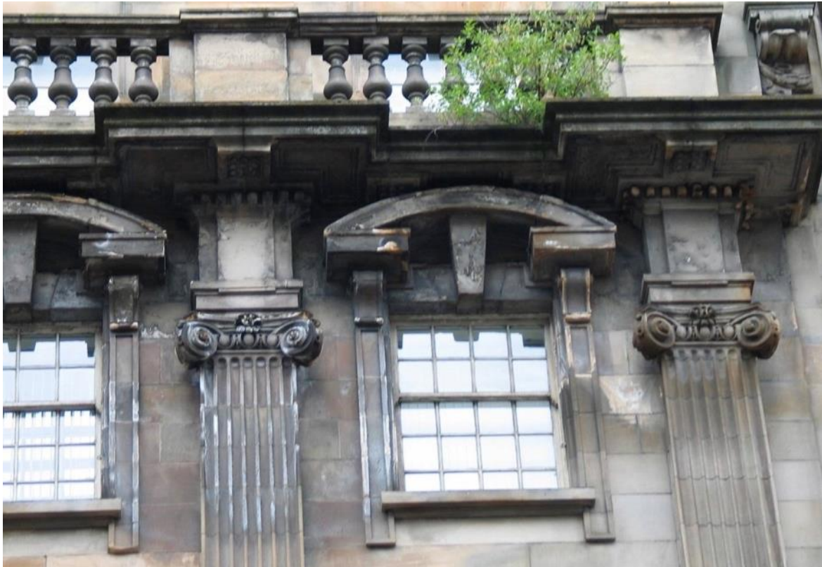
Glasgow: Evidence of a long-standing water penetration failure
