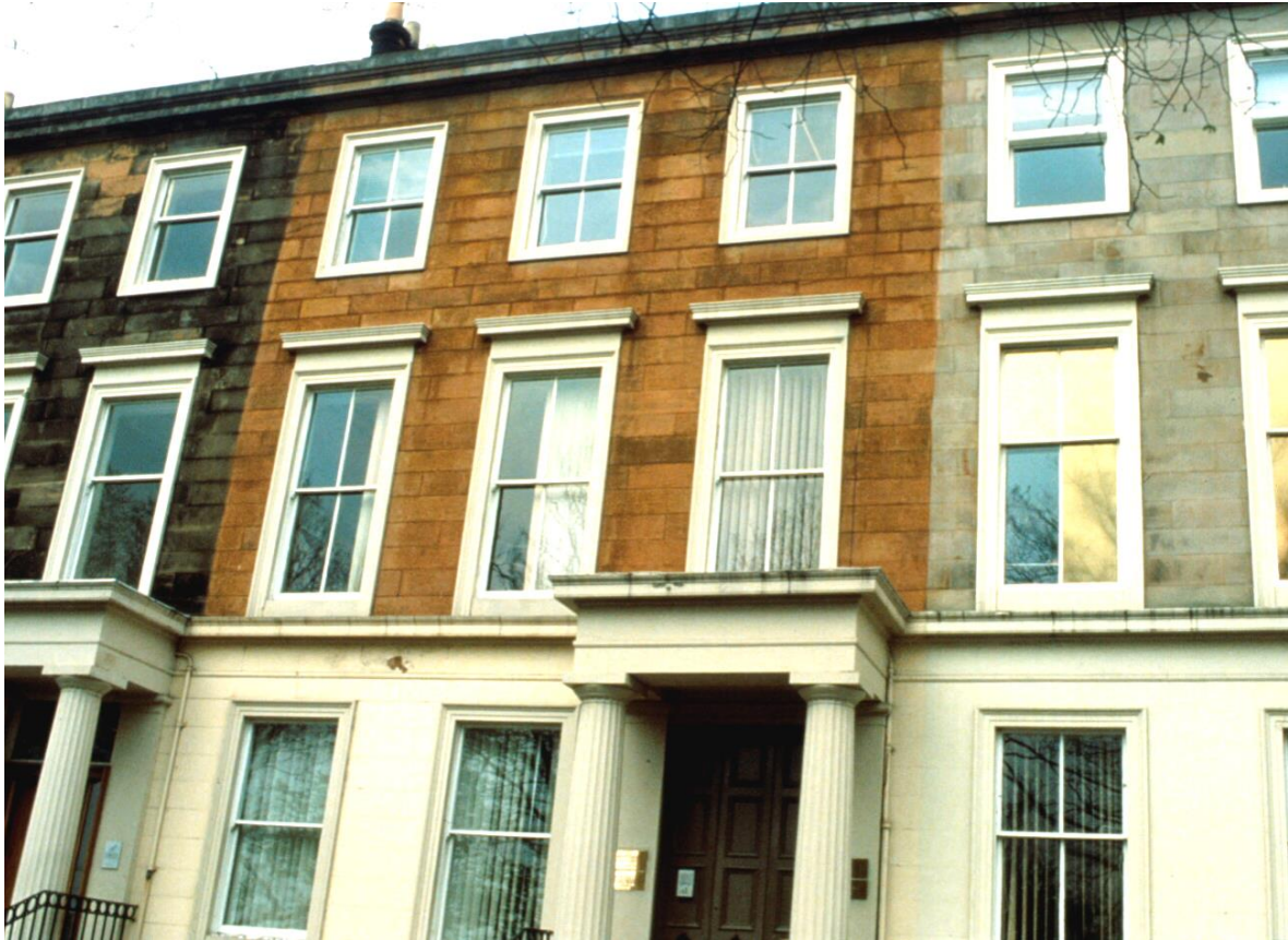
Glasgow: Ineffective control of different cleaning techniques
