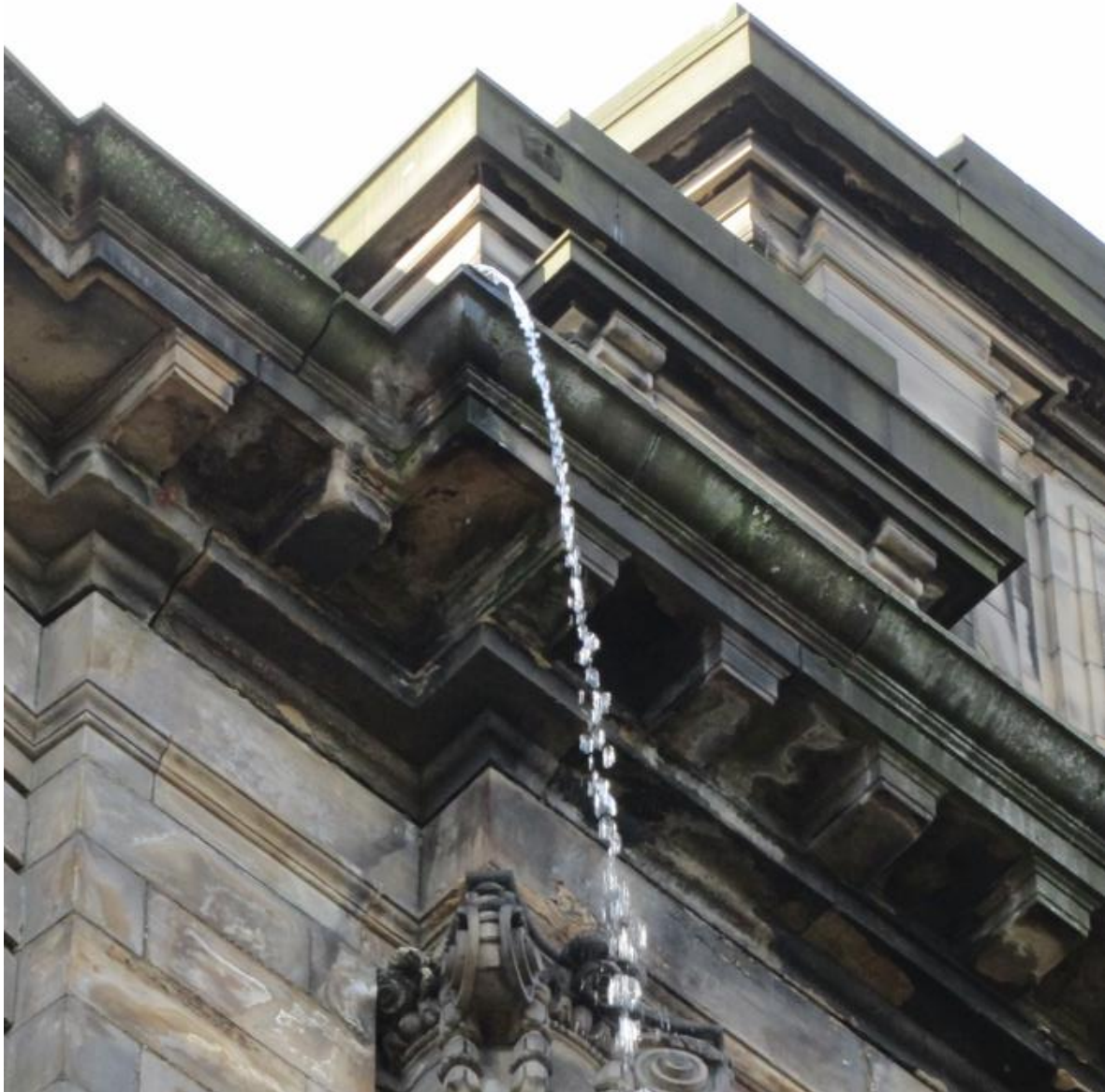
Glasgow: An obvious consequence of ineffective monitoring and maintenance
