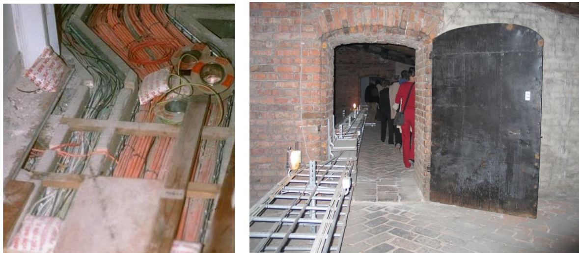
Services installations can create complexities in maintaining fire compartmentation
