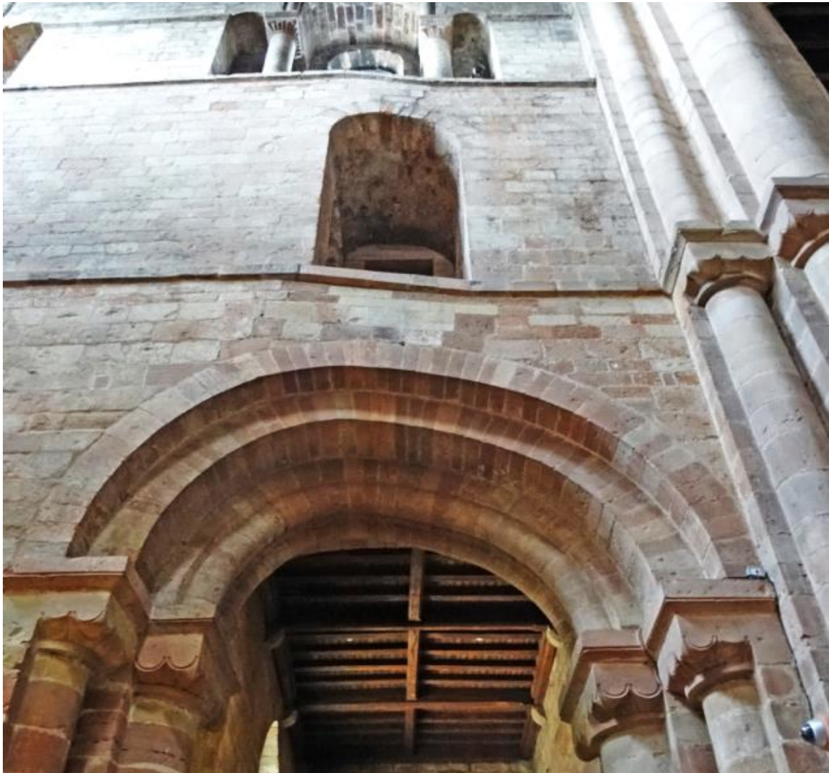
Carlisle Cathedral: Structural distortion DSC04902a June 2022
