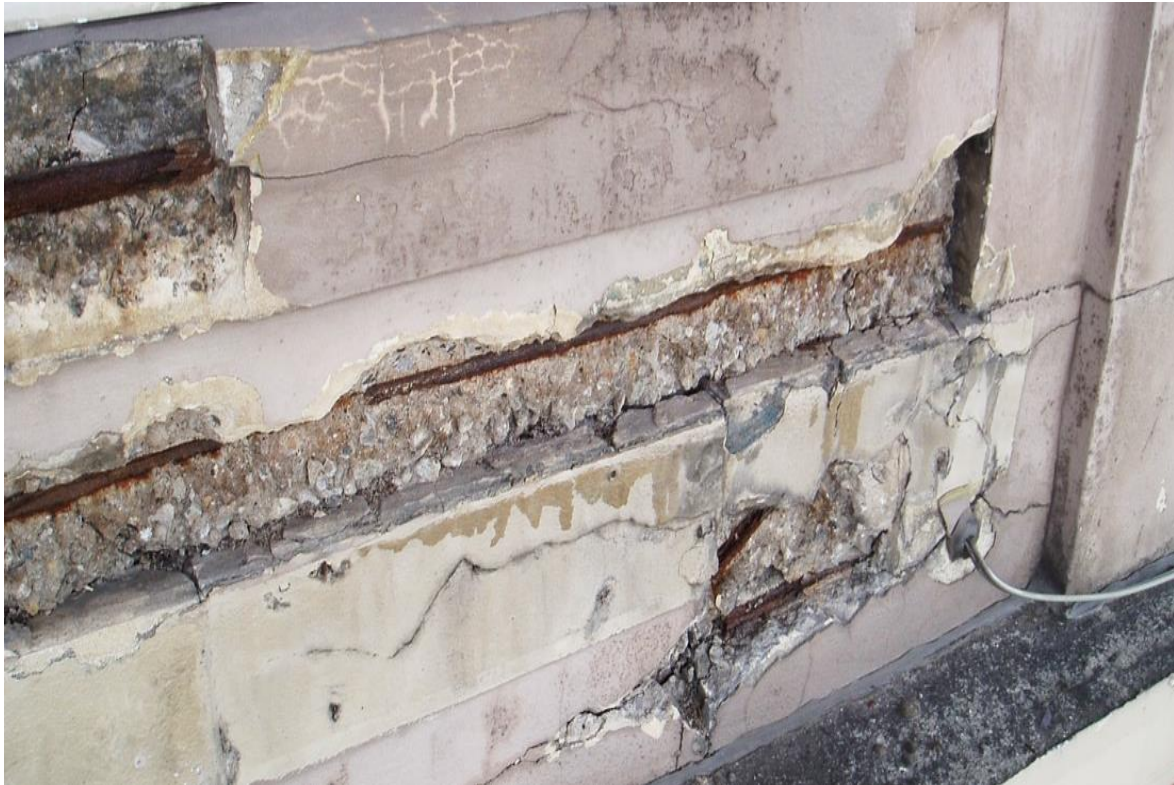
Insufficiently covered rusting-steel induced concrete cracking and spalling
