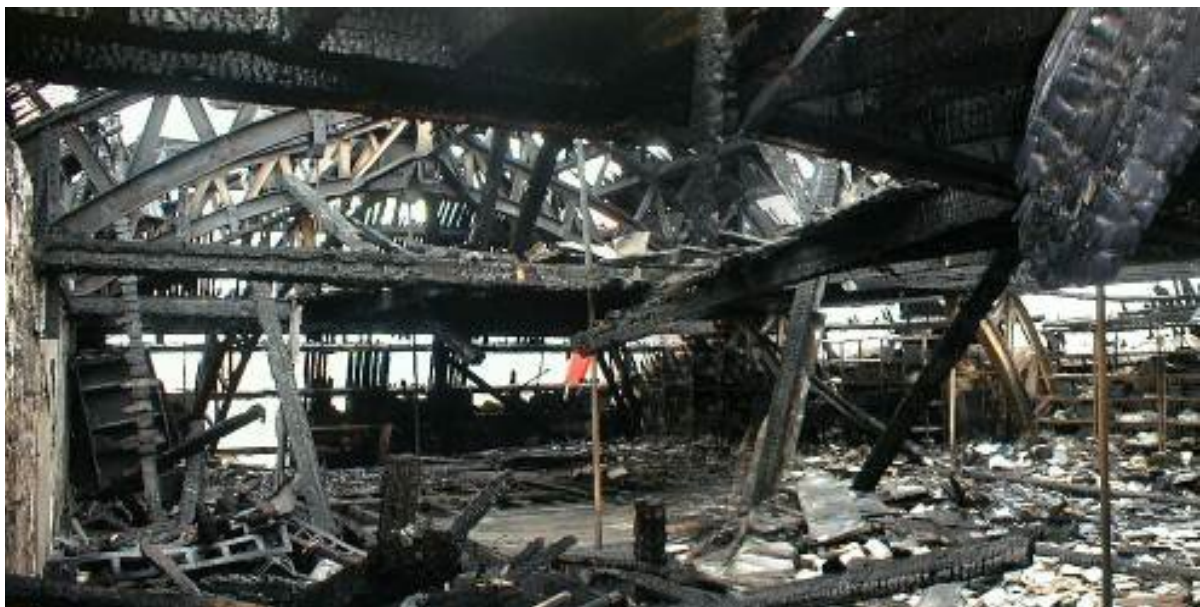
University of Lyon Library 1999: Post-fire interior
