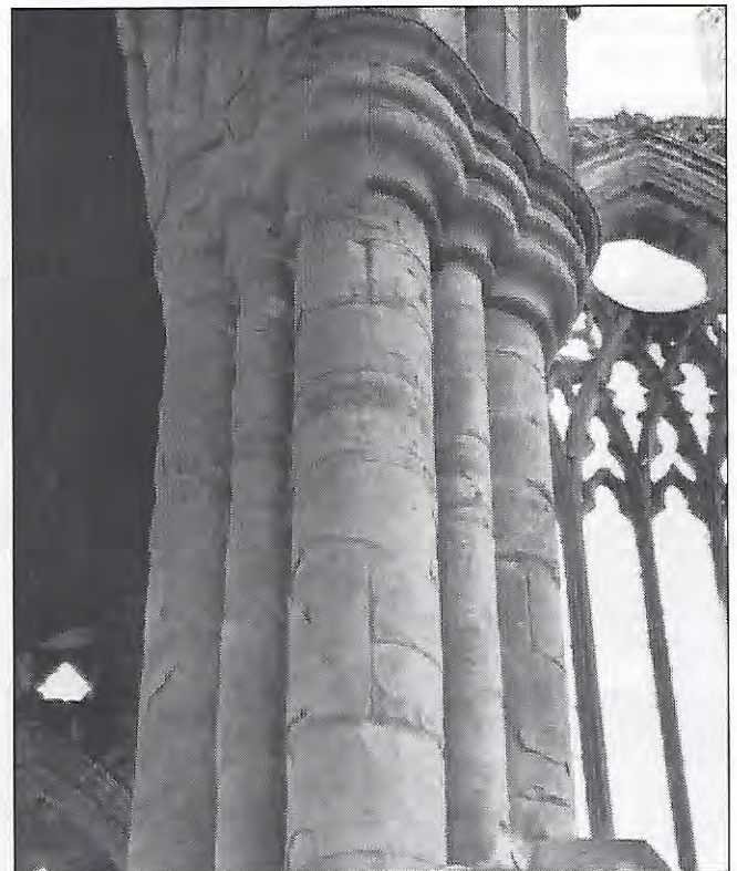
Problems with contour scaling at Tintern Abbey
