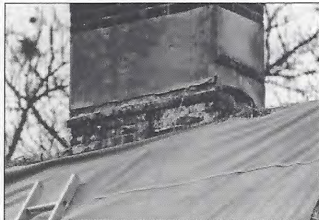
Long straw is cleaned back to sound material before the application of a new "spar coat" coat is applied. The crack in the chimney brick work requires repair before the thatch coat is completed.
