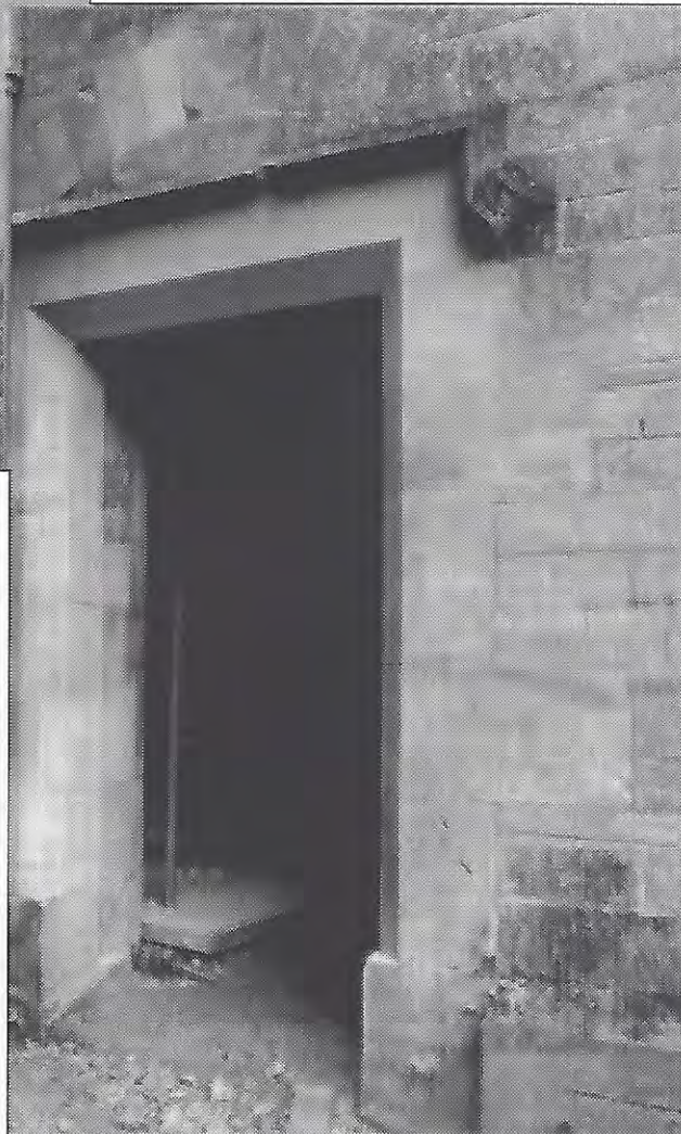
Laundry doorway, 1995 training project with Weymouth College. Above: the Laundry door before repair. Below: after repair. Photographs: Margaret Lister.
