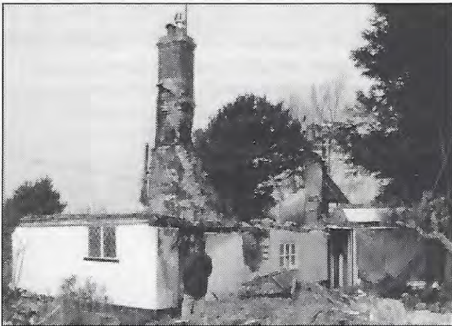
Both these chimneys are faulty. The fire started in the chimney in the foreground. A wood burning stove had produced heat so intense that the entire chimney had distorted and cracked.
