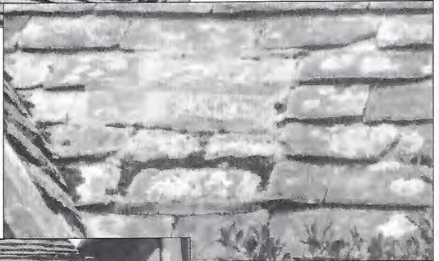
A sorry repair on a magnificent medieval Church
