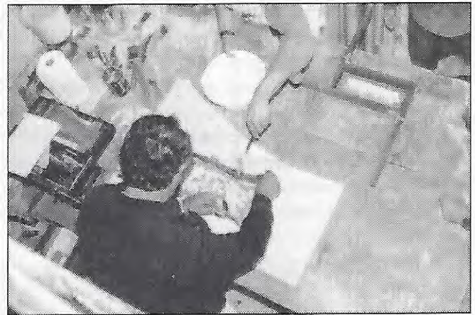
Instructors Andrew Ladygo and Rory Brennen prepare to make a mould from an existing section of plaster ornament for repairs to a decorative cornice.
