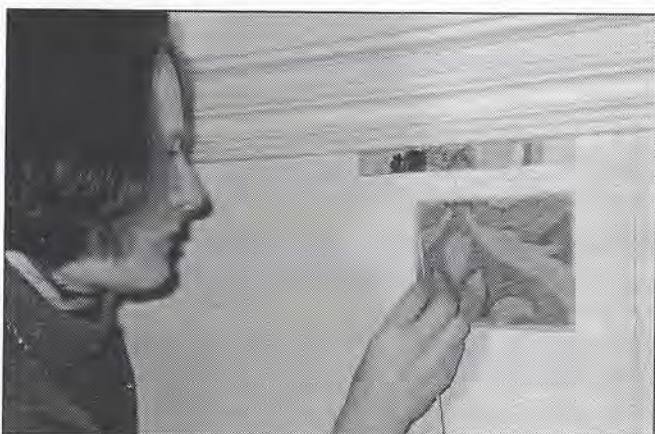
Paint removal to reveal original wall decoration in Coffee Lounge at St Pancras Chambers.
