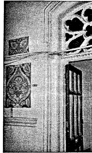
Original fanlight and door in first floor corridor adjacent to exposed stencil work. See previous page.
