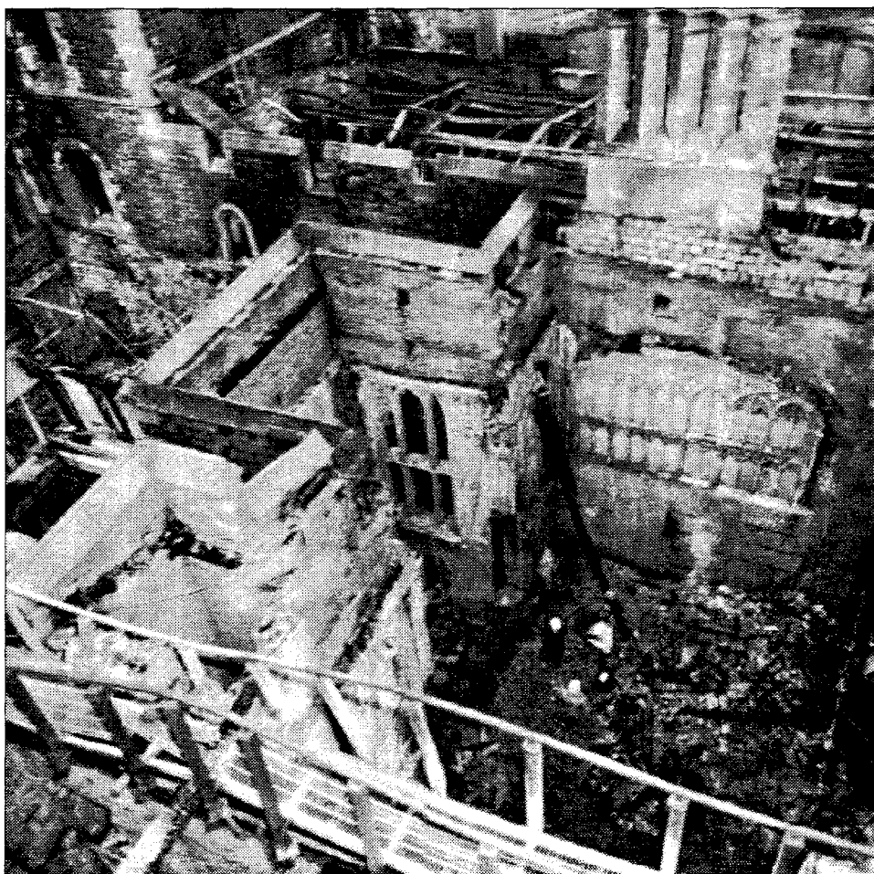
Figure 2 Fire damage at Windsor Castle
